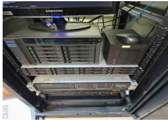
Vista general Datacenter 2025
