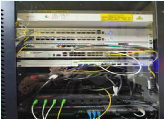
Firewall Fortinet instalado
